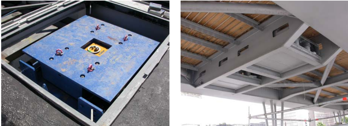
Figure 6-2: Examples of installed TMDs
