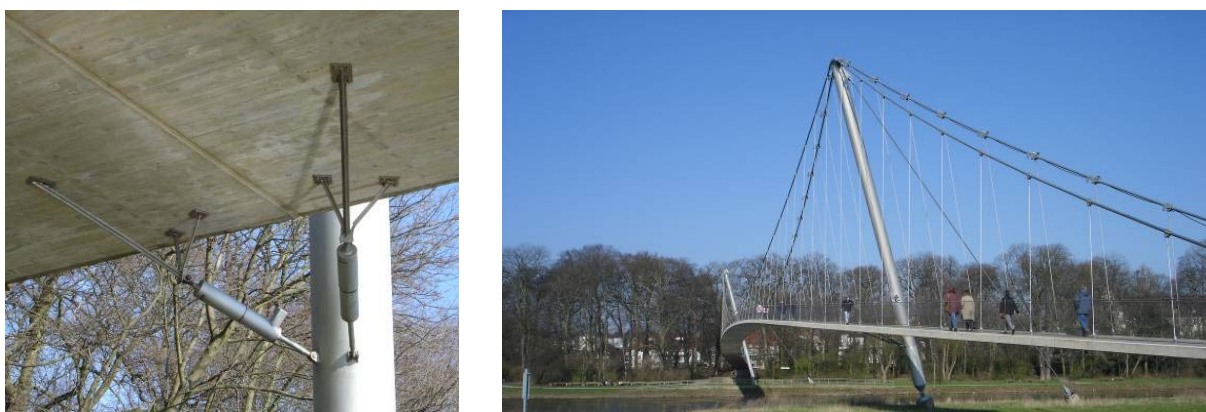
Figure 6-1: An example of installed viscous dampers
